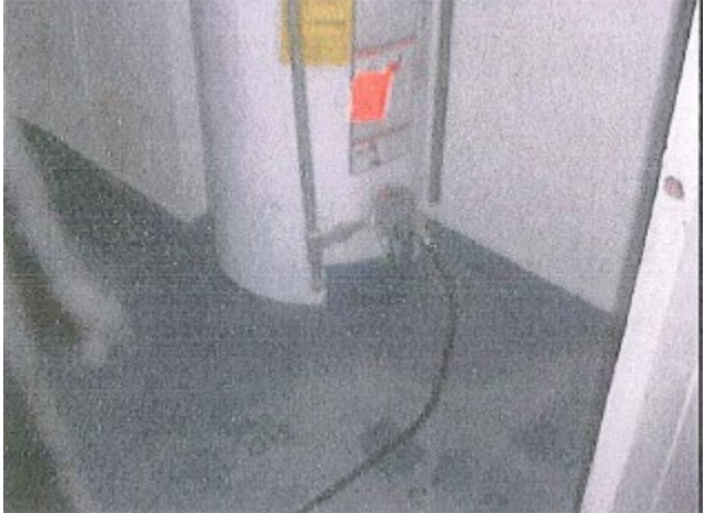
Draining Water heater
