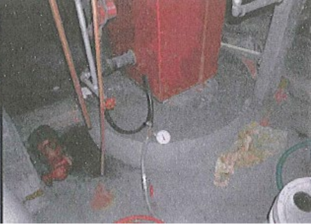
Boiler During Pressure Test
