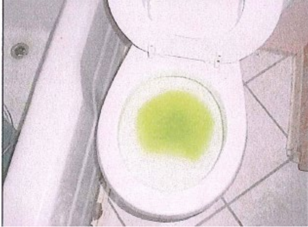
Example of Incorrect Anti-Freeze
